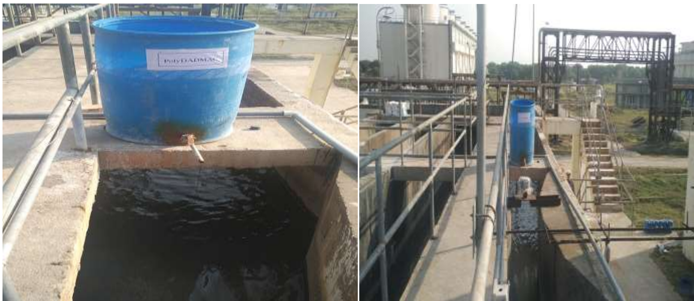
PolyDADMAC dosing in CW Clarifier inlet channel
