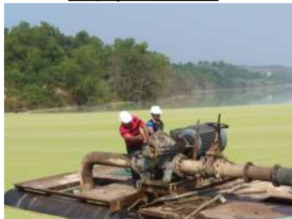
Pumping of return water
