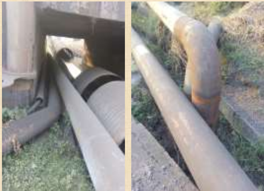
Over lapping of pipes
