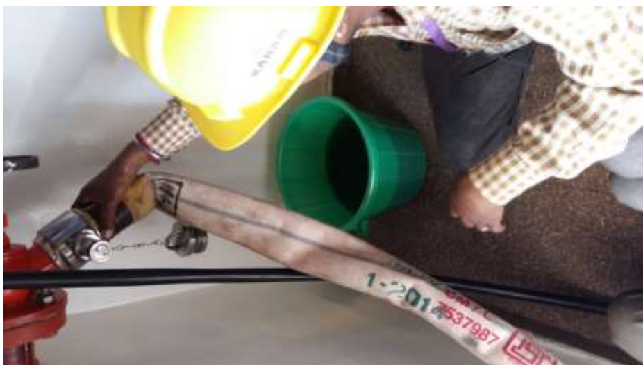
Fig. 20: Black Coloured water from Fire Hydrant due to SRB
