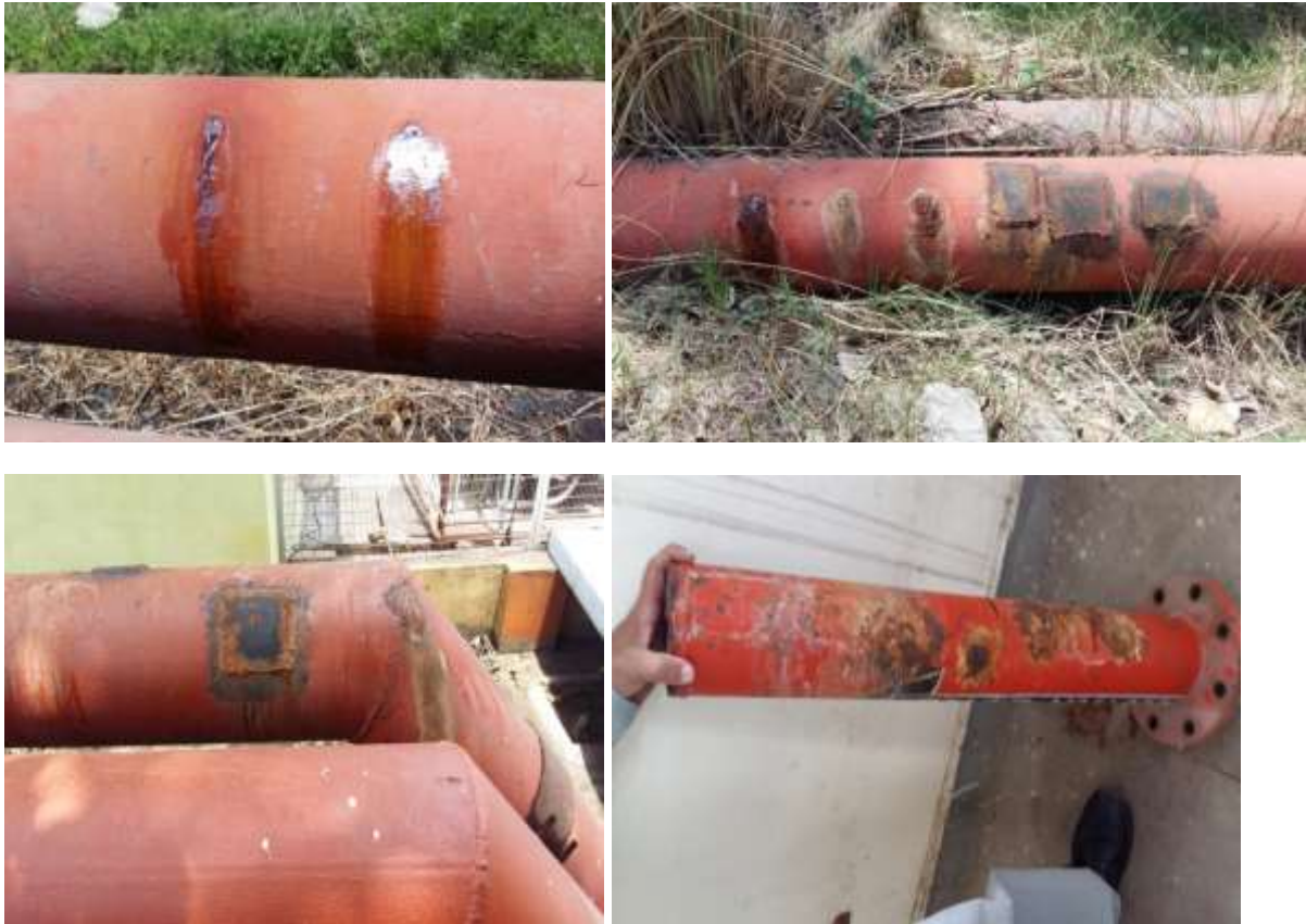
Fig. 15 to 18: Typical Failures in Fire Water System
