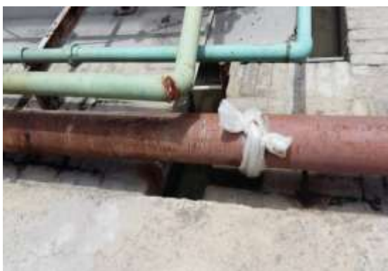
Fig. 9: Leak in service water pipe
