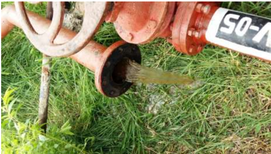
Fig. 19: Dark brown coloured fire water due to Biofouling
