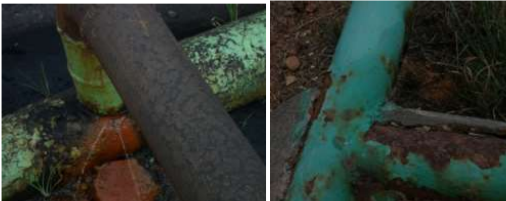
Fig. 7 & 8: Severely Corroded Service Water Pipelines
