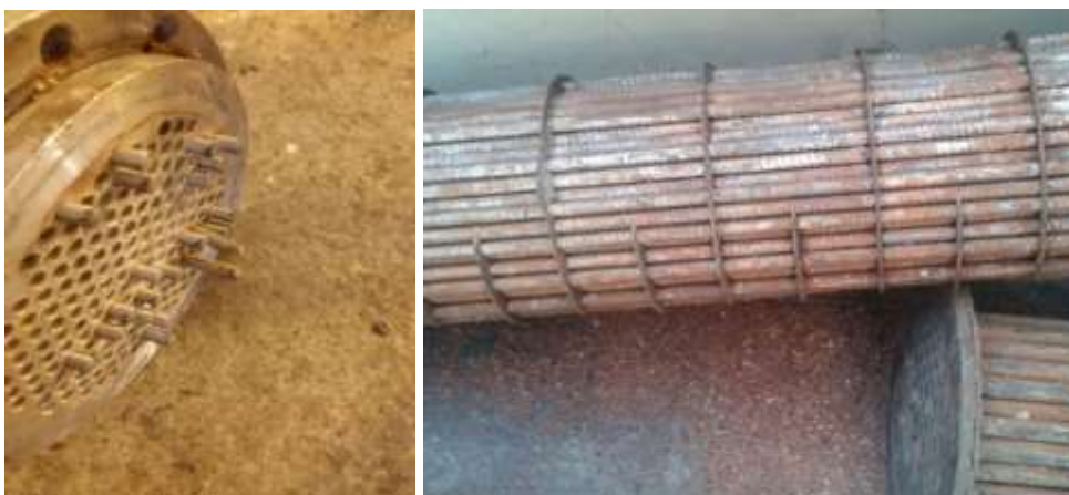
Fig. 3 & 4: Plugged Heat Exchanger Tubes and Corrosion and Fouling on external surfaces of Tubes (Corrosion due to Service Water)
