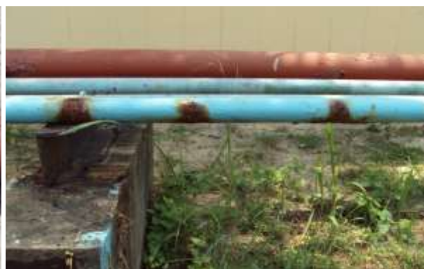
Fig. 10: Corroded service water pipes
