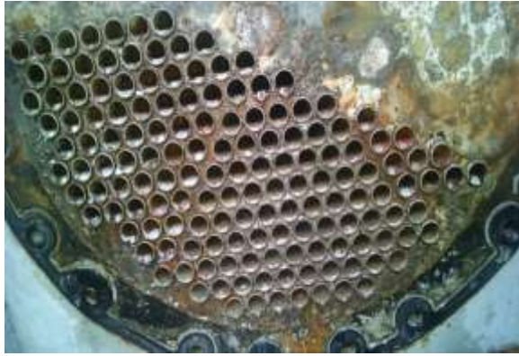
Fig. 12: Severe Biofouling, MIC, Deposition on Cooler Tube Plate
