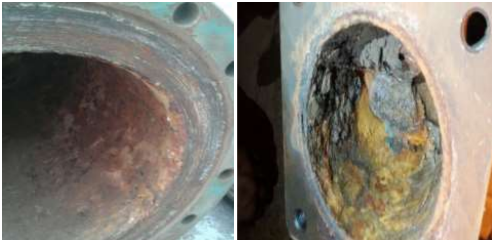
Fig. 1 and 2: Severely corroded inner surface of Heat Exchanger Shell and Water Boxes
