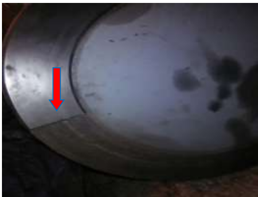
Damaged valve wedge of MS valve
