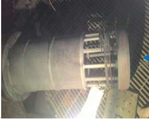
Damaged MS Strainers-RHS
