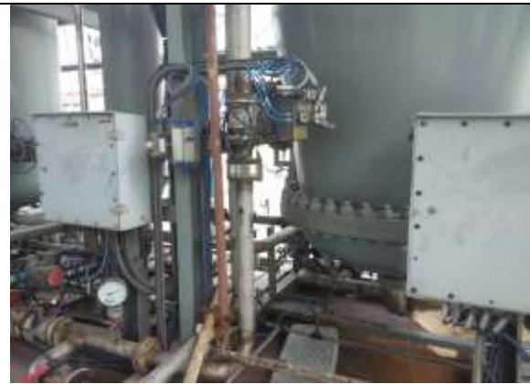
ANION REGNERATION UNIT
