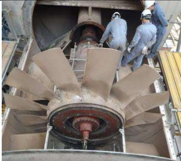
Noise Level sensor mounting on Booster Fan
