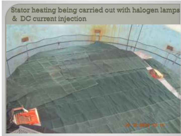
Figure-2: Dry out of stator with halogen lamps and DC current injection
